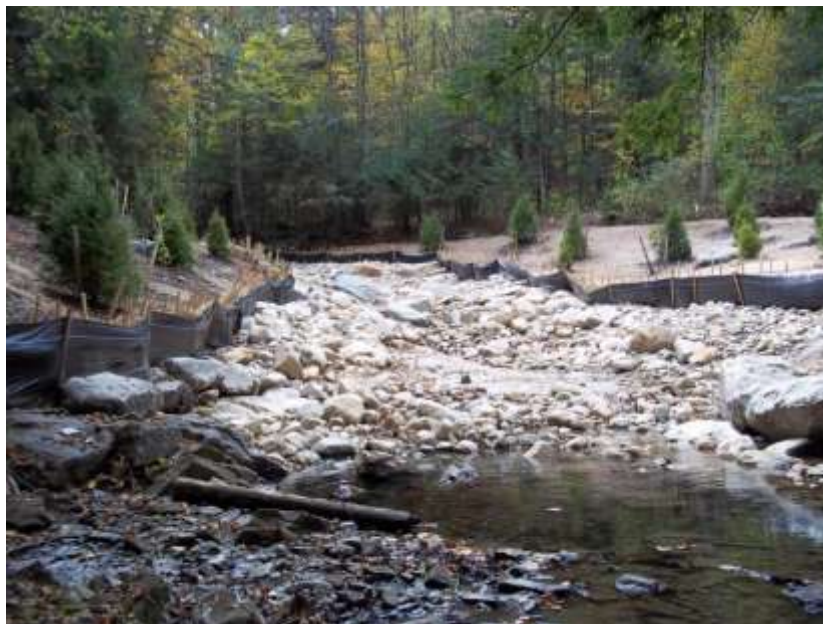
Hathaway Brook streambed near the end of restoration activities (Photo credit: City of Pittsfield)
