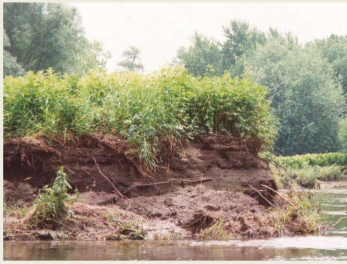
Bank Failure and Erosion Puts PCBs into the River over Time
